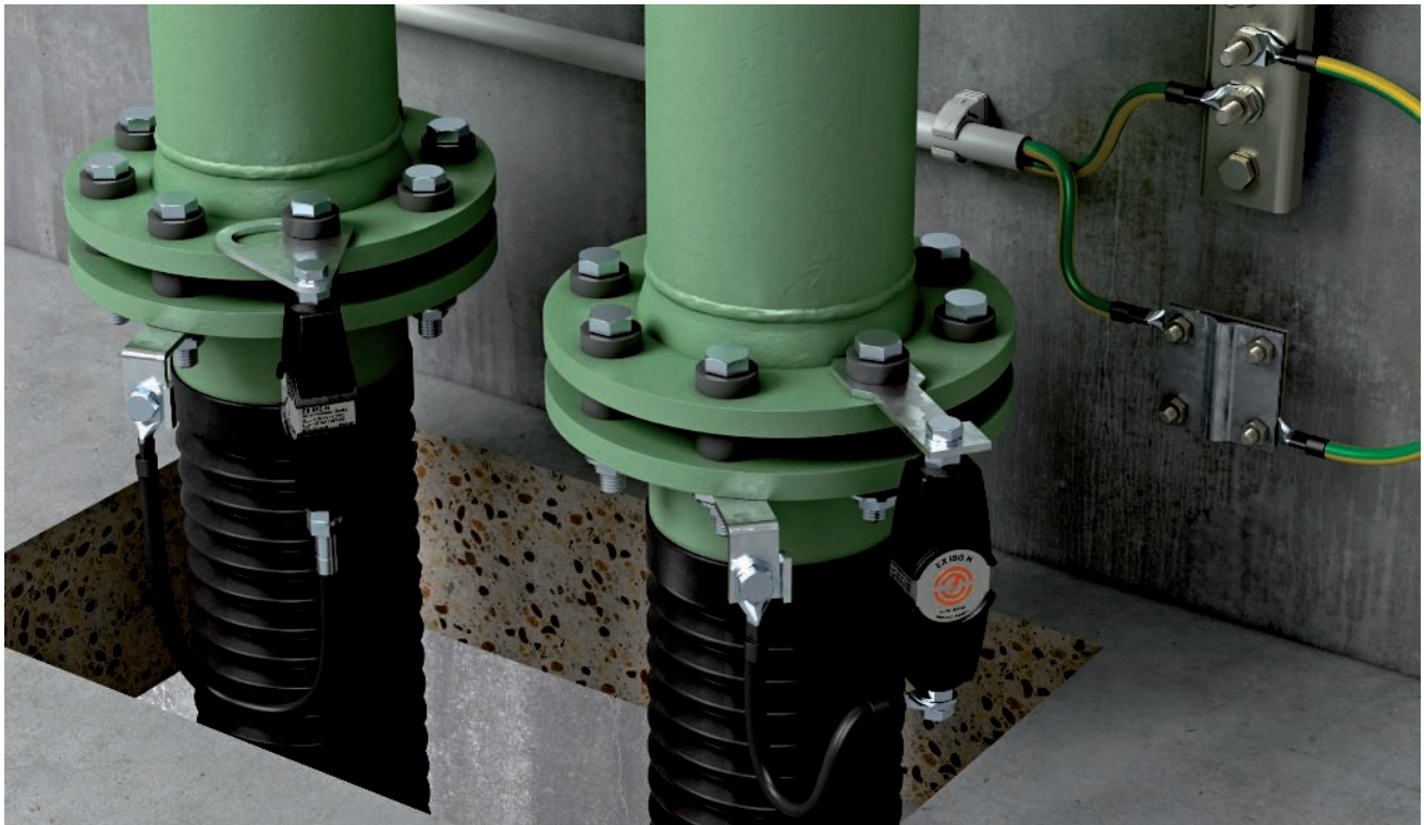
Spark gap mounted on insulating sections
